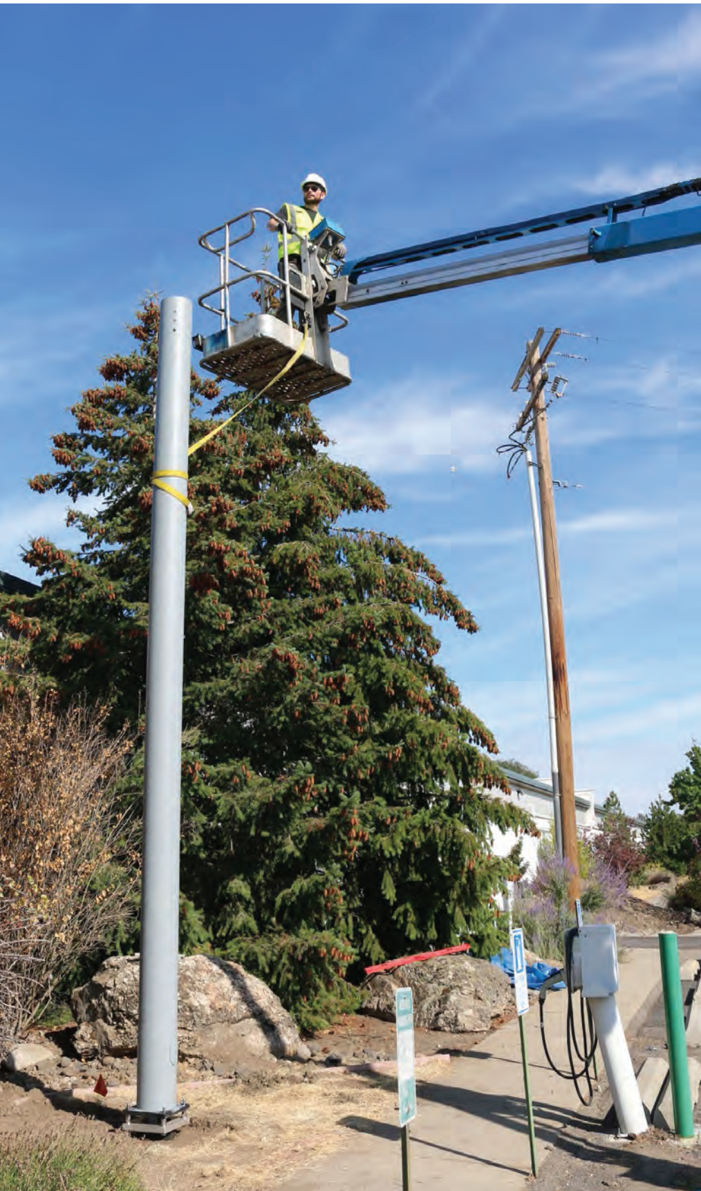
EasyStreet Systems team members installing a fiber composite pole in rural Bay County, Florida. EasyStreet Systems
