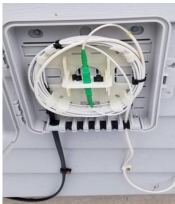
Figure 2 Baseline TAP Box Installation
